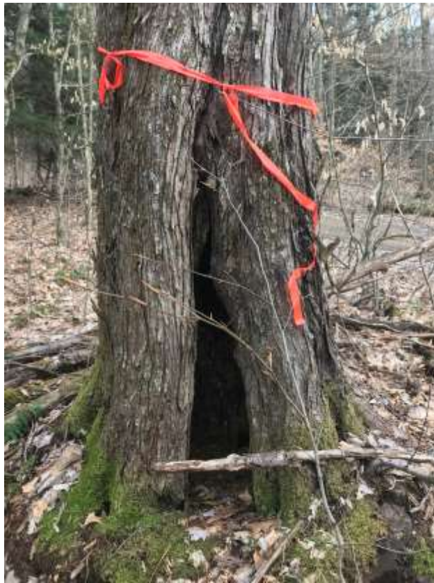
However, from the other side, you can see that it is overgrown and decayed. It now has no timber value.
